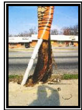
Figure 3. West view of the struck pole.
