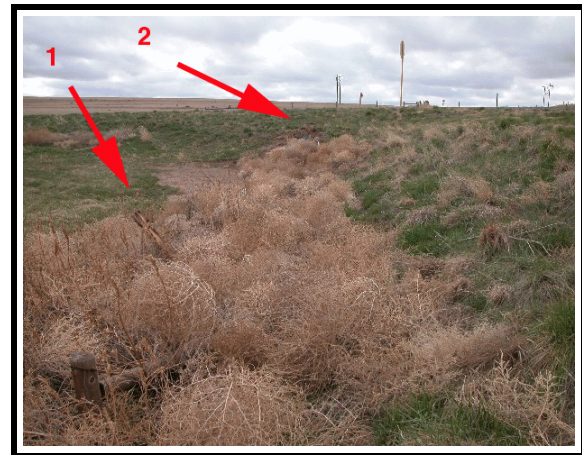
Figure 3. Impact with post, then culvert
