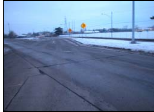
Figure 4. Northbound view of initial area of impact.
