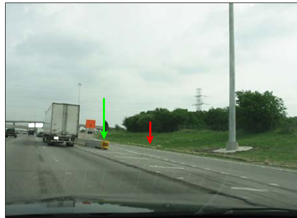
Figure 1: Overview of exit lane and impact attenuator at the end of the gore (green arrow), the impact attenuator has been repaired, red arrow shows police reported area of case vehicle's final rest
