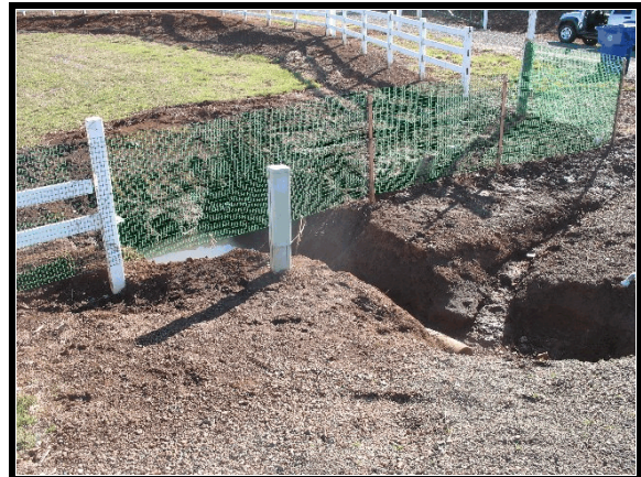
Figure 4. Side view of sink hole (east)
