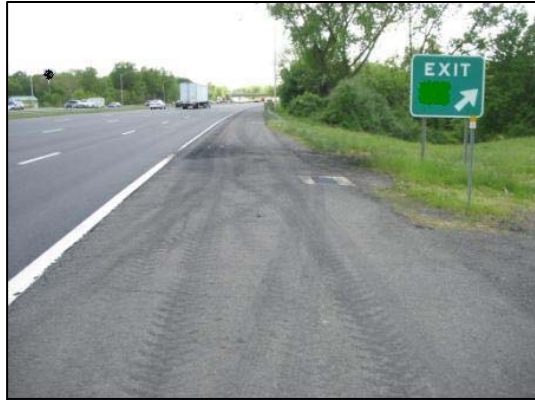
Figure 3. Area of the fire on the right shoulder of the interstate.
