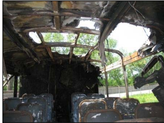
Figure 9. Burn-through and sag of the roof and roof structure of the motorcoach.
