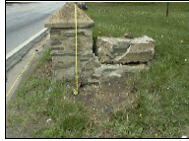
Figure 2- View of the stone wall struck by the front of Vehicle #1
