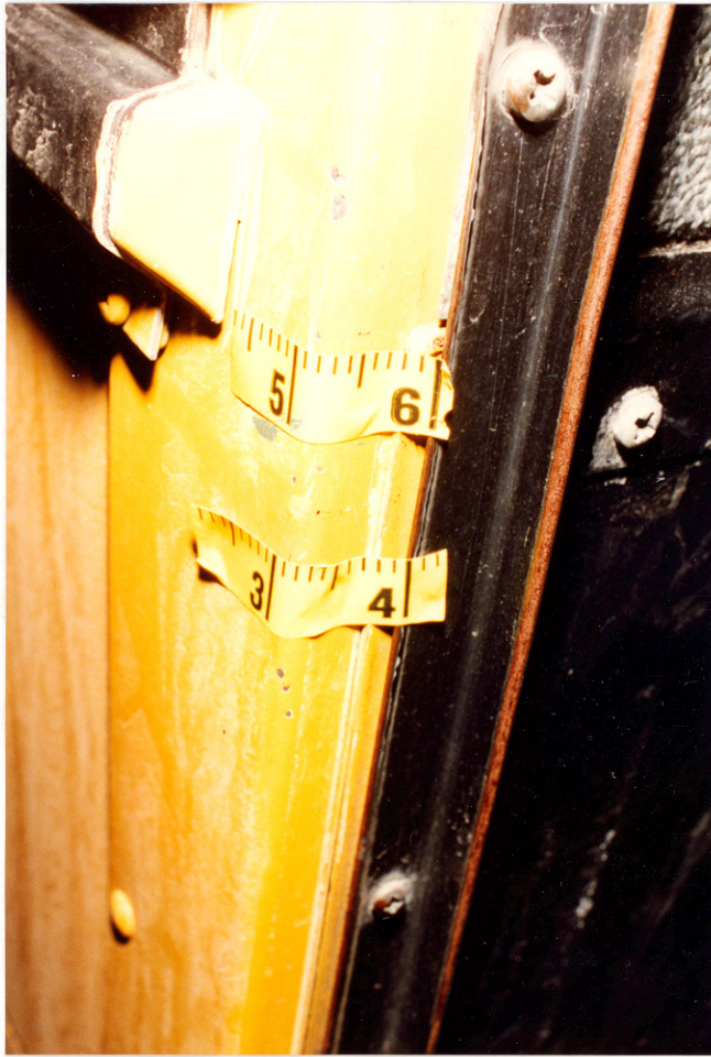
7. Paint abrasion from draw string contact on the rearward edge of the door opening.
