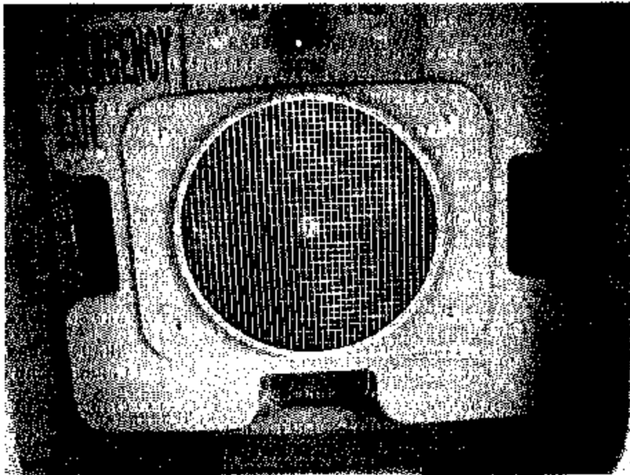
Photograph 10 - Emergency Roof Exit Label
