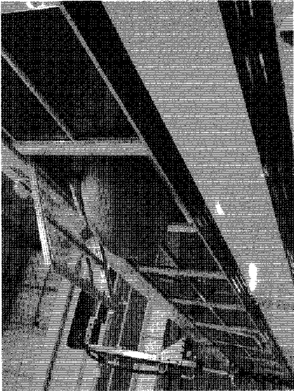
RF Exit Opened After Roof Loading is Attained with Measuring Device in Place
