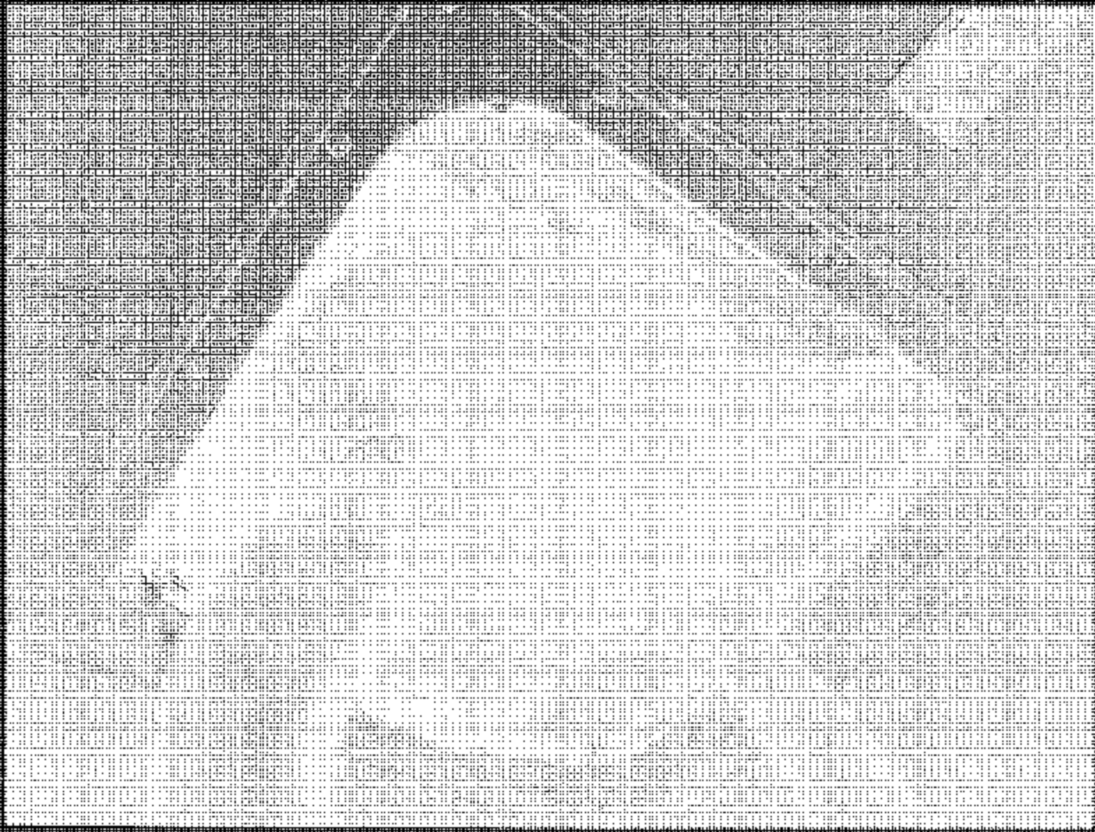
Roof Exit Edge-to-Edge Clearance
