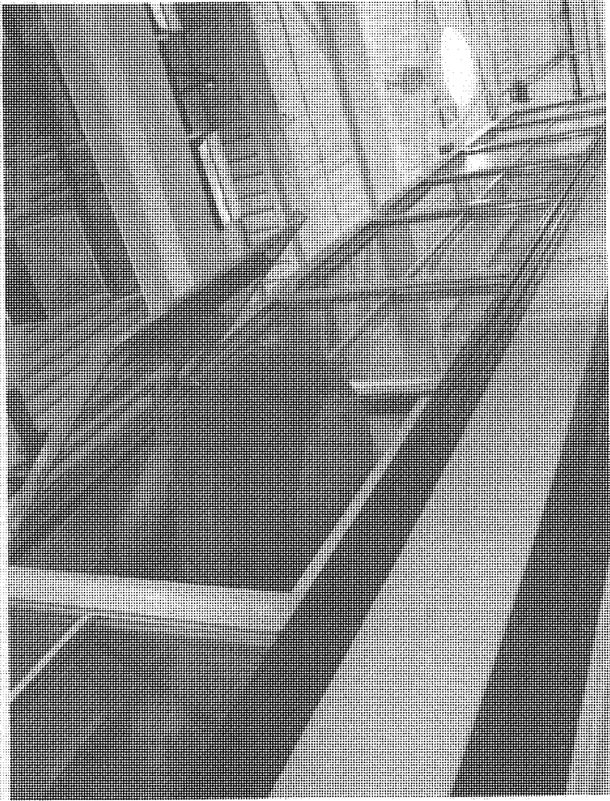
LF Exit Opened After Roof Loading is Aligned with Measuring Device in Place
