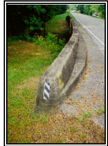
Figure 2. Struck concrete bridge railing.
