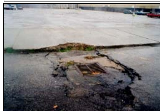
Figure 3. Close up of the depressed sewer collector
