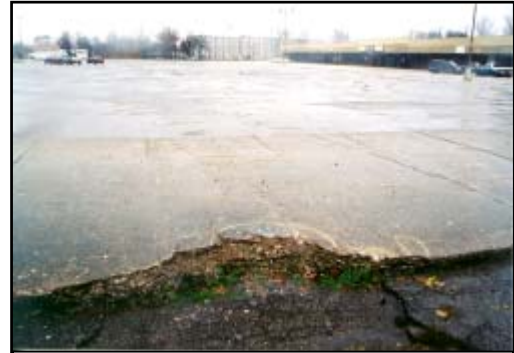
Figure 5. Close-up of concrete curb edge at impact point
