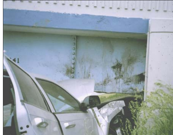
Figure 9: Police on-scene photo showing impact impression to steel bridge support beam
