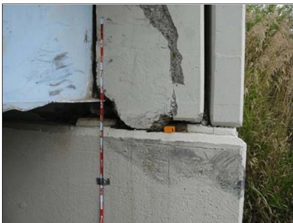
Figure 7: Arrow shows right front wheel impact to overpass bridge abutment, measurement rod graduated in tenths of meter
