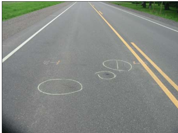
Figure 3: View north to impact gouges in southbound lane
