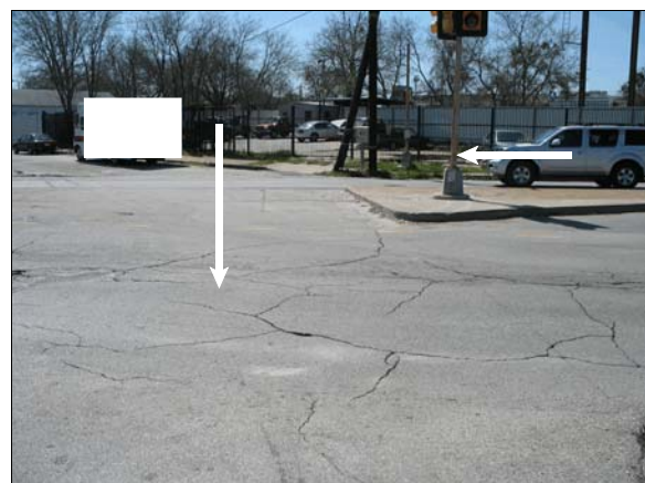
Figure 4: Left arrow shows impact area in intersection (view from Toyota's path of travel); right arrow shows impacted traffic signal pole
