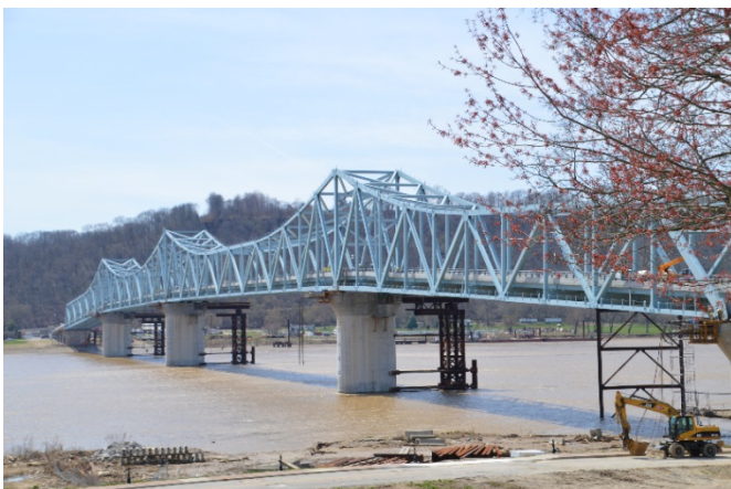
The bridge after the slide was completed. (Courtesy of FHWA Indiana Division Office)
